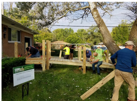
Staff of The National Bank of Indianapolis build an accessibility ramp through Servants at Work Inc.
